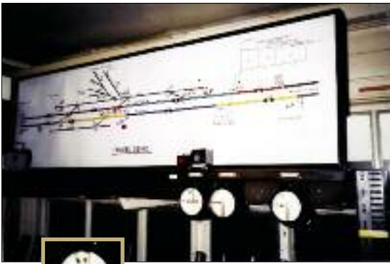
Repeater signal for calling-on arm (left-most instrument), Forders Sidings (note: rest of signalbox equipment not designated)
