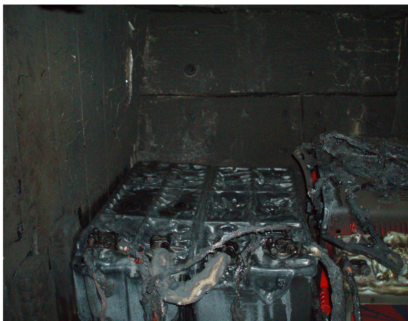
Seat of the fire in the battery bank cables connections
