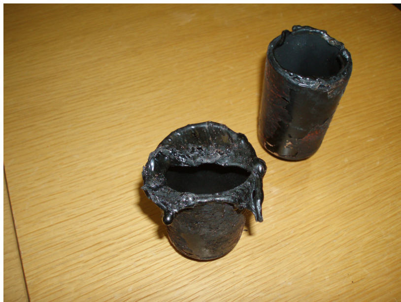
Melted plastic CO 2 discharge nozzle
