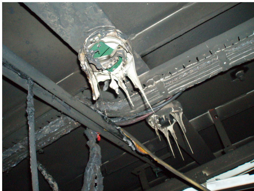
Melted fire detectors
