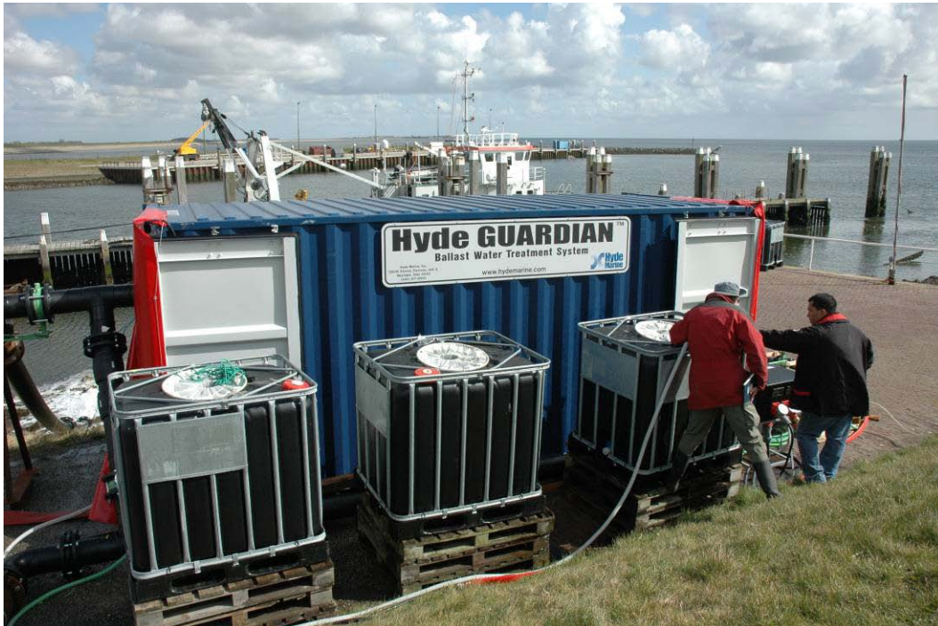
Figure 10: overview of the Hyde-Guardian™- Ballast Water Treatment System in the NIOZ harbour. In front of the container are the three IBCs with the 50 µm inline sampling nets.
