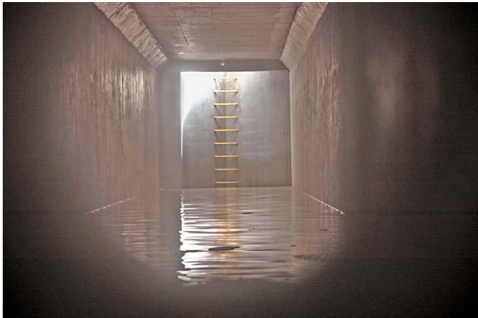
Figure 2: Inside view of one of three subterranean water tanks
