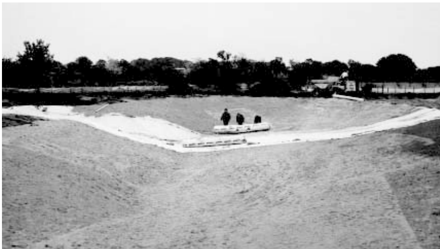
Plate 4 Lining large waterbodies requires detailed design and installation with natural materials to protect and disguise them
