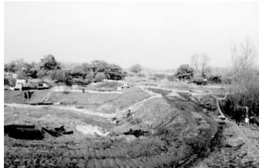
Plate 2 Construction sites can become a jigsaw of ecological treatments prior to the main works and requiring equally diligent supervision
